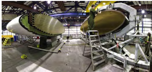
Figure 2.12: Radar array inside dome structure [21]
