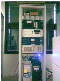
Figure 1. Photograph of the servers’ room
