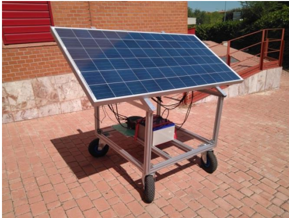
Figure 17. Photovoltaic system seen from the front.
