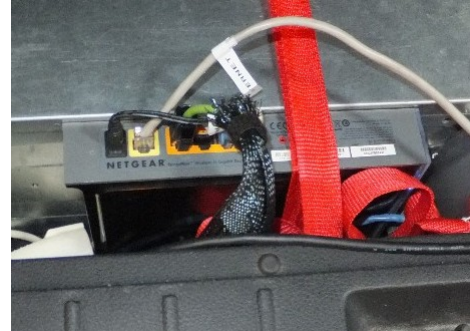
(b) Ethernet switch for sensors and TESLA
