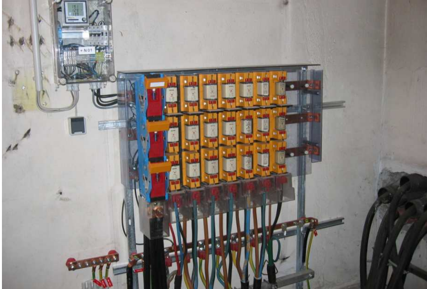
Figure 31: "Substation Low Voltage part" Source: Stadtwerke Düsseldorf
