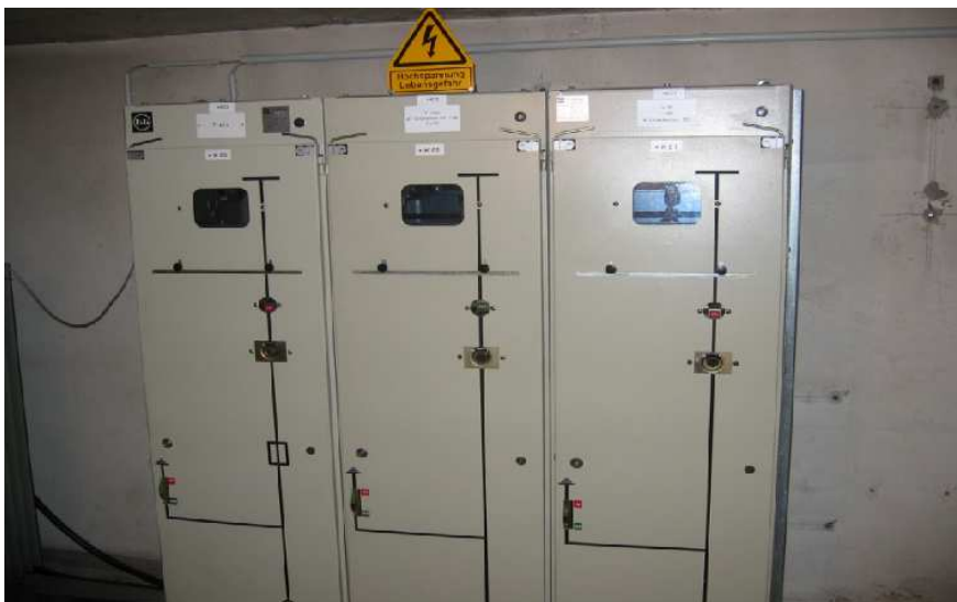
Figure 32: "Substation Medium Voltage part" Source: Stadtwerke Düsseldorf
