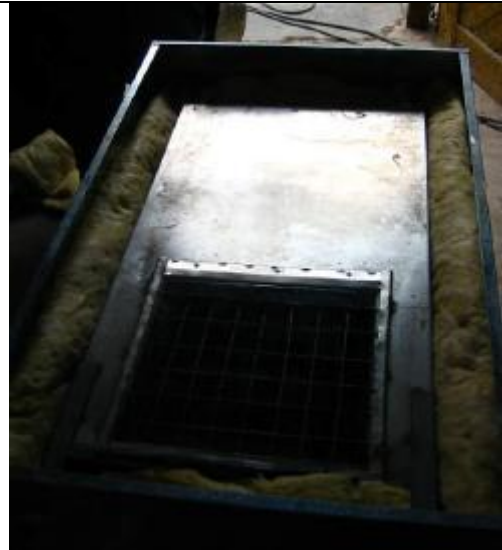
After all parts are finished the oven can be insulated with mineral or rock wool. The spacing between inner and outer wall is 10 cm. All in all 8 m 2 of mineral wool is needed.
